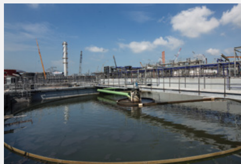
One of Sembcorp's wastewater treatment facilities on Jurong Island
