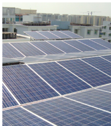
Solar panels installed atop HDB blocks
