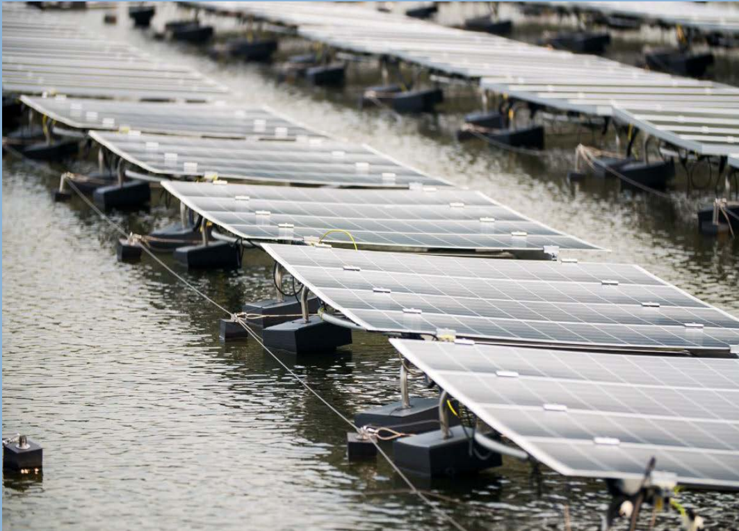
FLOATING SOLAR PANELS AT RESERVOIRS
