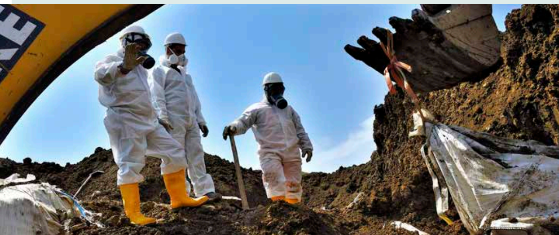
EXCAVATION OF POPs PESTICIDES AT THE LAGLUJA PESTICIDE BURIAL SITE IN GEORGIA. PHOTO BY VLADIMIR VALISHVILI.
