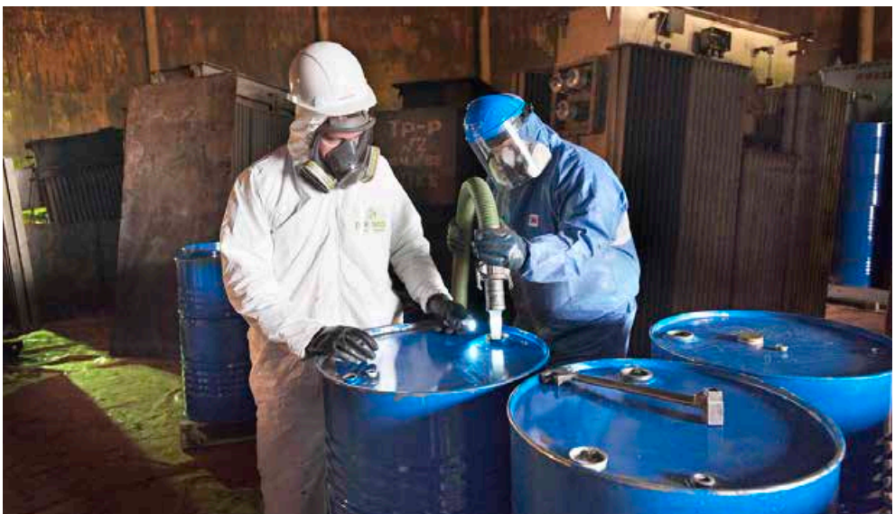
DRAINING OF PCB OIL FROM TRANSFORMERS AT ARCELORMITTAL TEMIRTAU IN KAZAKHSTAN. PHOTO BY POLYECO.
