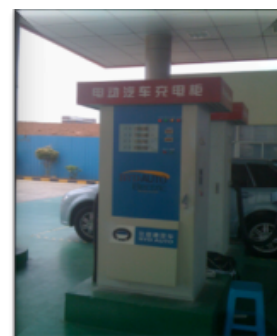
Fig B2: 180 kW Fast Charger at BYD in Shenzhen
