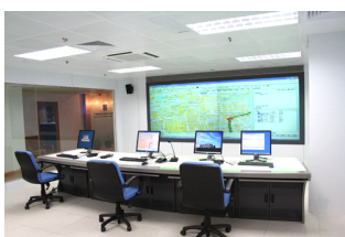
GPS monitor center
